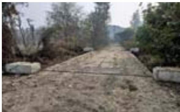
Figure 75: Abandoned approach in Rajau Paraspur SWM Plant
