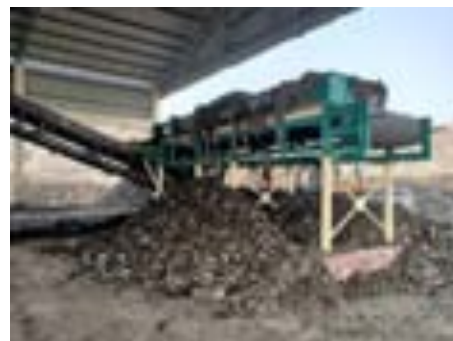
Figure 77: Treatment facility in Bakarganj SWM plant
